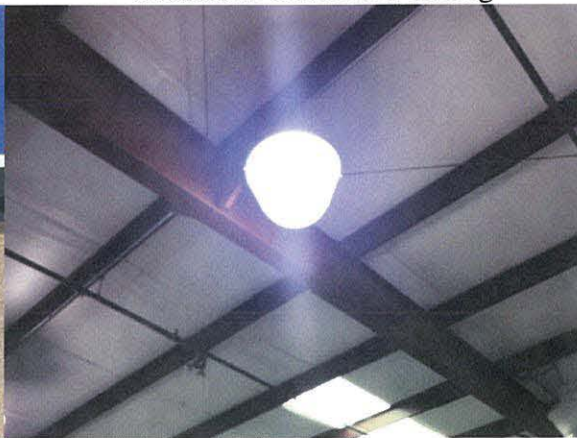
Warehouse/Indoor Storage Lighting
