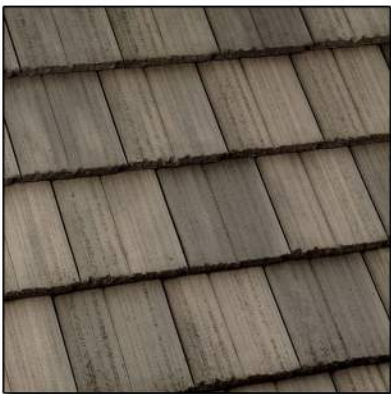
Roof Mfg: Eagle Roofing Double Eagle Ponderosa 987 Brown Gray Range
