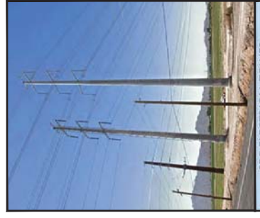
SRP ELECTRICAL TOWER
